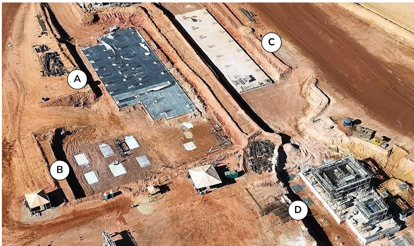
Figure 2: Civil works underway on the Tucumã Project's future process plant, including (A) rougher and cleaner flotation cells, (B) Jameson cells, (C) pyrite flotation, and (D) ball mill (July 2023).
