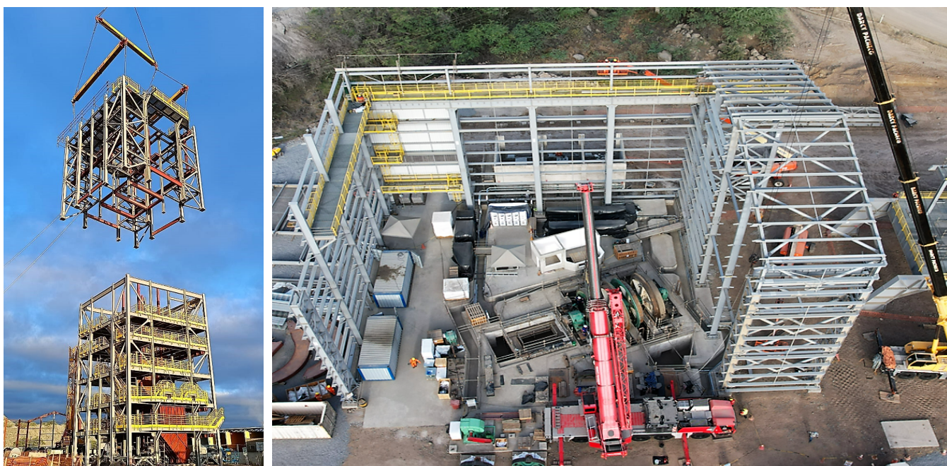
Figure 5: Hoisting of pre-assembled headframe at the Caraíba Operations' new external shaft in July 2023 (left). Figure 6: Construction and assembly of the personnel and material winder building as of July 2023 (right).
