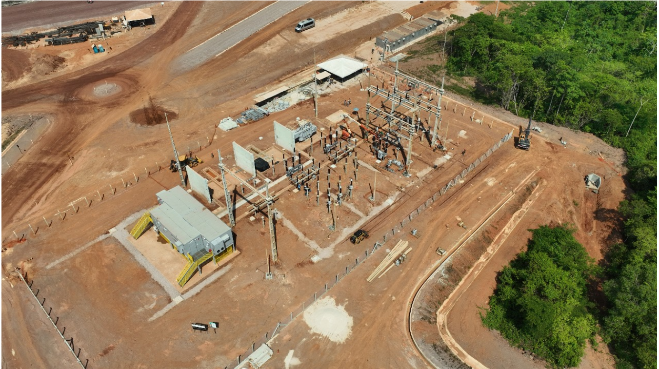
Figure 6: Electrical substation prepared for final tie-in to the national grid.
