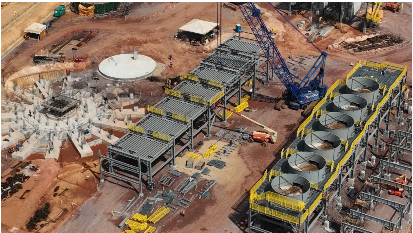
Figure 3: Flotation cells and tailings thickener foundation.
