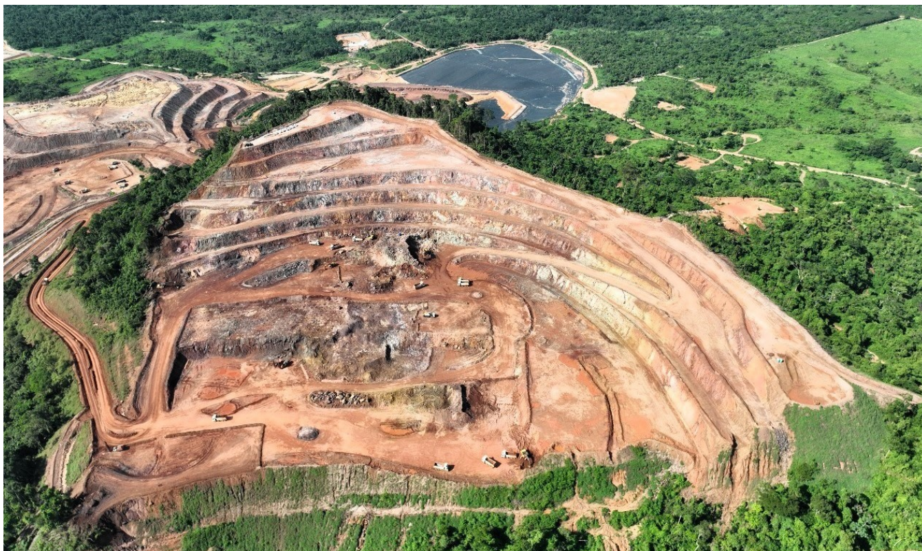
Figure 1: January 2024 aerial view of advanced pre-stripping activities, which are 10% ahead of schedule and tracking towards completion at the end of Q1 2024.
