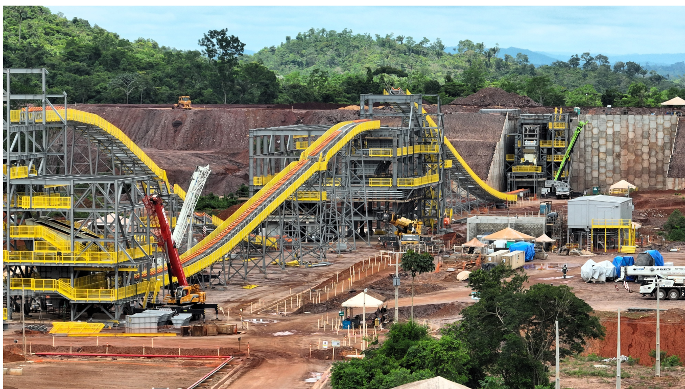
Figure 4: Primary and secondary crushing, screening and conveyance systems.
