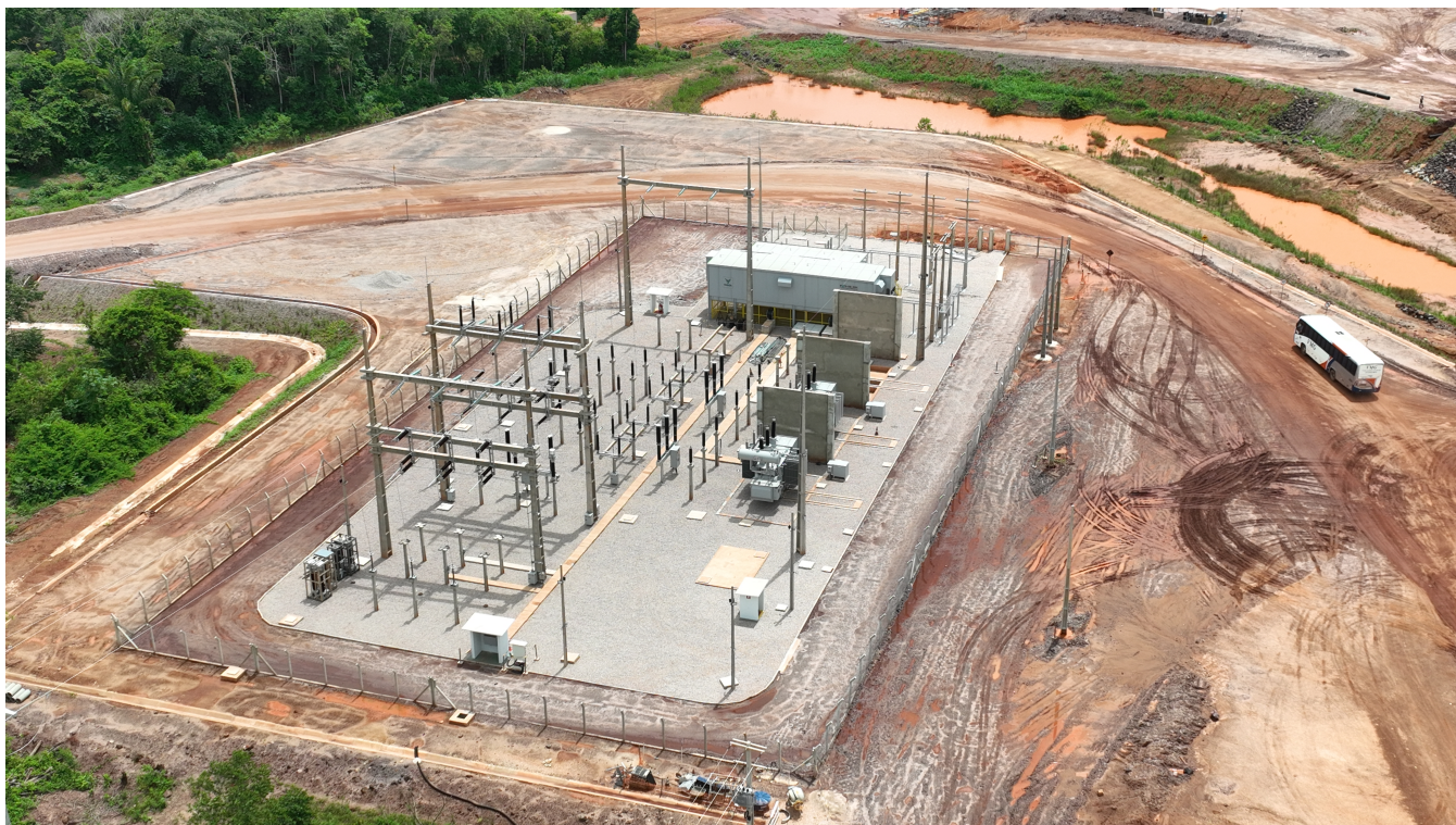
Figure 5: Completed primary sub-station and power line with tie-in to the national grid as of January 2024.
