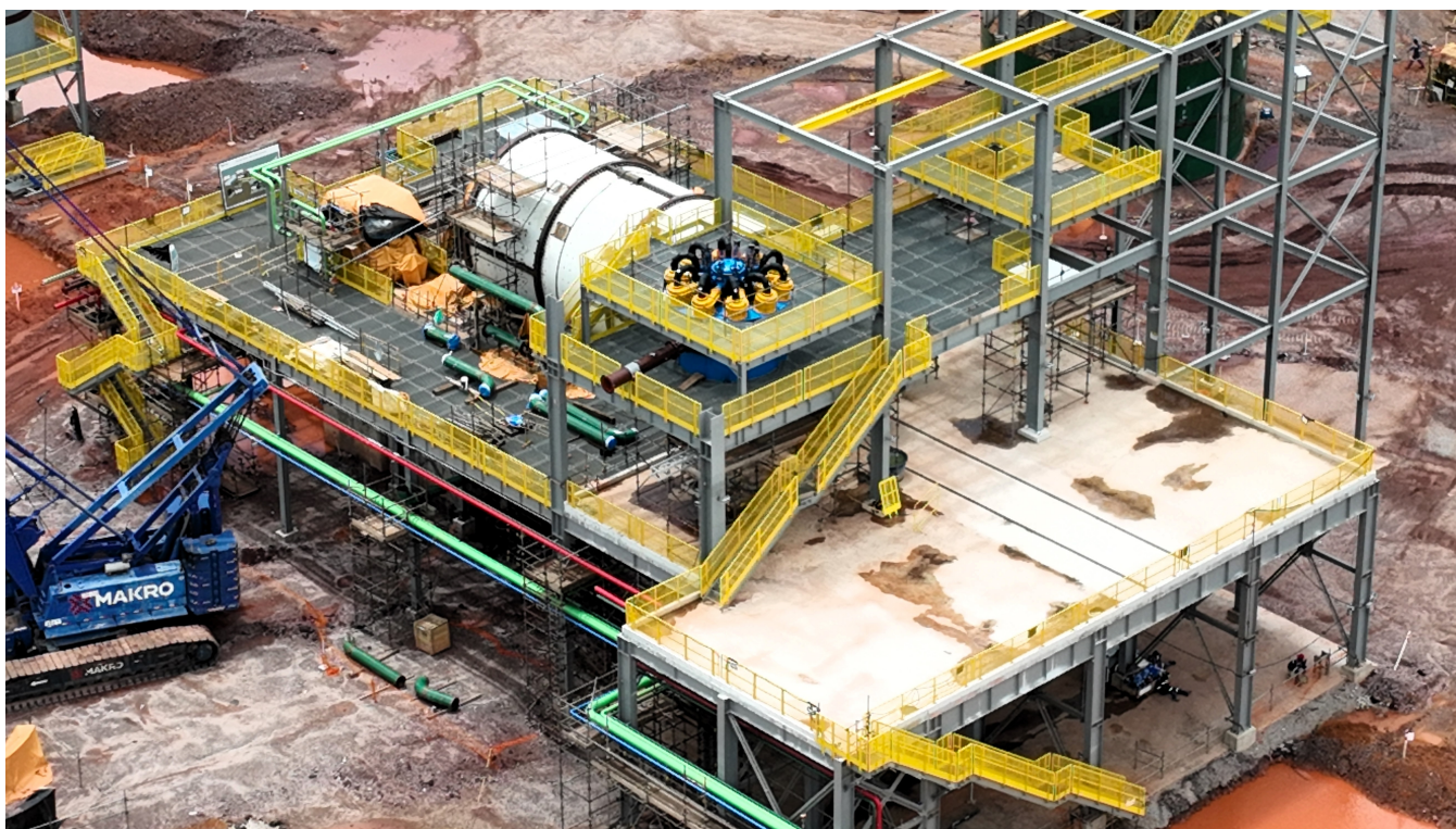
Figure 2: Ball mill and hydrocyclone battery as of January 2024.
