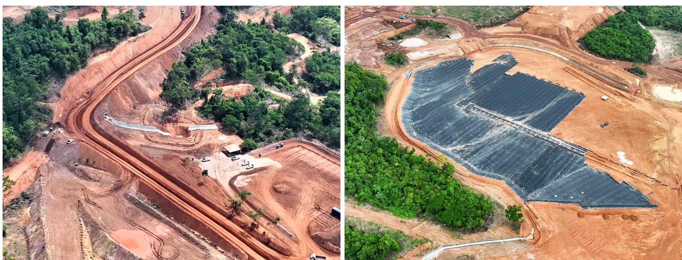
Figure 2: Tucumã Project mine access road and completed drainage infrastructure (left) and waste rock dump with installation of HDPE liner underway in October 2022 (right).
